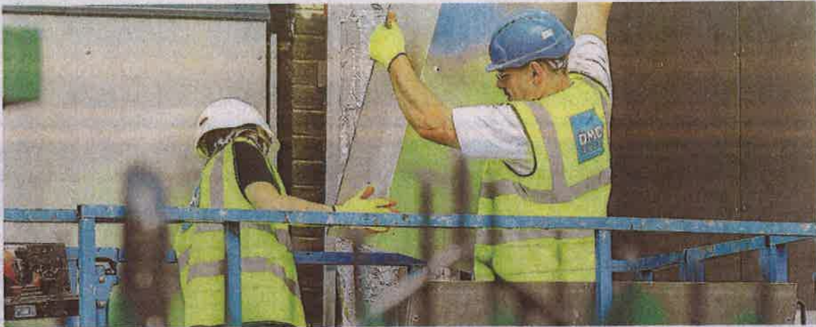
Some insurers have imposed exclusions in professional indemnity cover over non-compliant cladding. PHOTO: AP
